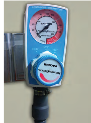
Fig. 2.10: Testing vacuum in operating room using vacuum gauge.
